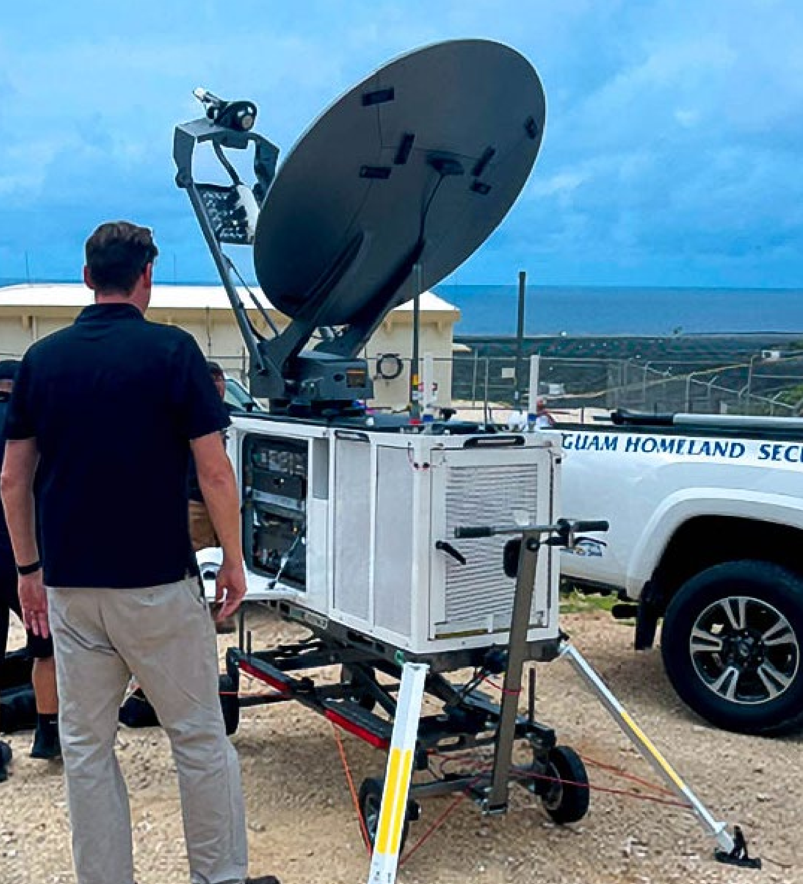
In order to validate and verify the initial buildout of the FirstNet network, the FirstNet Authority team traveled across U.S. states and territories, including Guam, as seen pictured, to ensure contract milestones were met.
